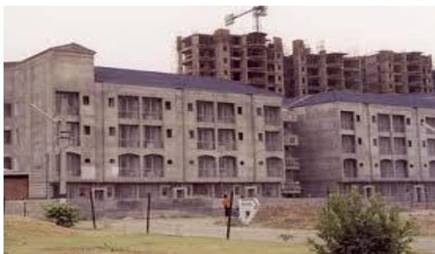
Illustration - "B" – Reinforced CLC Load bearing walls used for 4-storey dwelling at South of Delhi – 1997.
